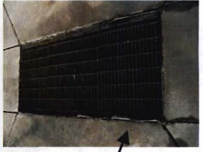
Floor drain in wash booth
